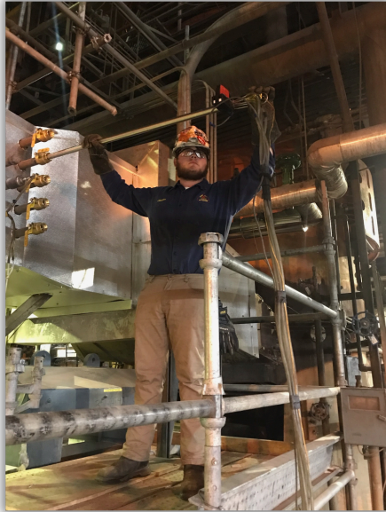
Figure 2: Storm team performing Primary Air Testing & Calibration
