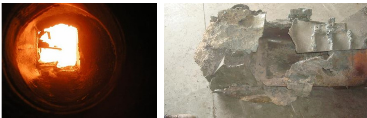
Figure 3: Burner damage from two sites with low airflow on damaged burner
