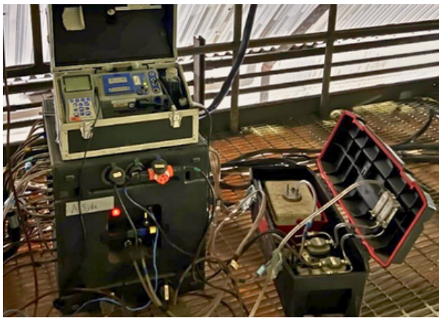
Figure 2: SOAR Equipment (PLC/Solenoid Box, Gas Analyzer & Gas Conditioner)
