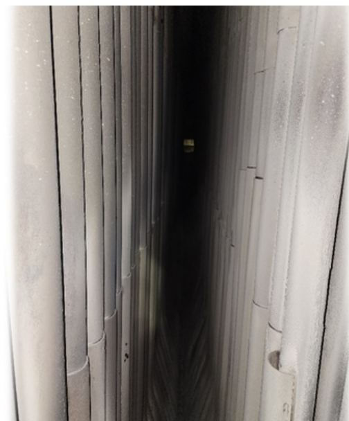
Figure 4: Generating Bank after 90+ days of operation (Much cleaner than before impulse cleaner)
