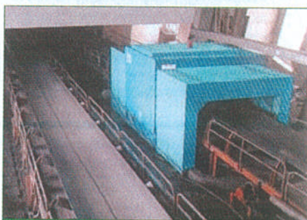
Figure 5. Sodern's Pulsed Fast and Thermal Neutron Activation (PFTNA) coal analyser.
