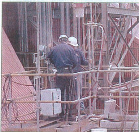
Figure 4. Insitu flyash sampling for representative flyash samples being collected during a boiler efficiency and comprehensive performance test.
