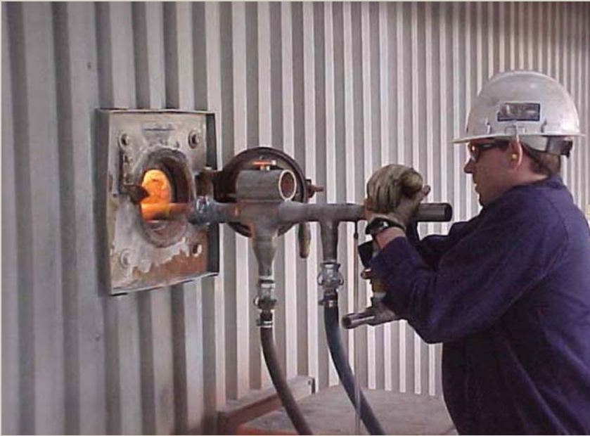
4. Testing, testing. A water-cooled, high-velocity thermocouple probe is used as part of a diagnostic test to quantify “oxygen rise,” furnace exit gas temperature, and flue gas composition stratification. Courtesy: Storm Technologies Inc.
