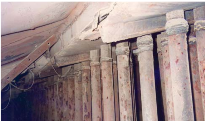
9. Air leaks. Leaks inside the nose arch (top) and casing (bottom) within the “dead air space” of a 1950s-vintage coal-fired boiler. Courtesy: Storm Technologies Inc.
