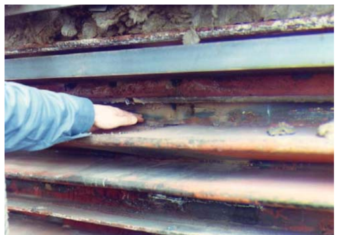
5. 15% loss. Leaks in an economizer expansion where the level of air in-leakage was about 15% that of total combustion air. Courtesy: Storm Technologies Inc.
