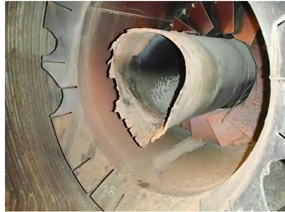
Figure 9: Damaged burner nozzle
