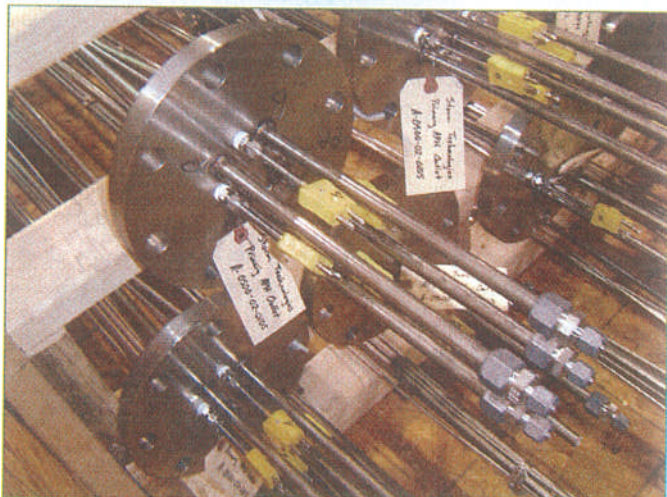
Figure 2. Multi-point flue gas sampling probes for boiler efficiency testing.
